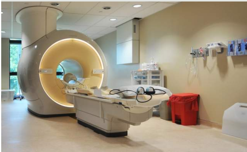
MRI Backup Cooling Jack C. Montgomery VAMC, Muskogee, OK
